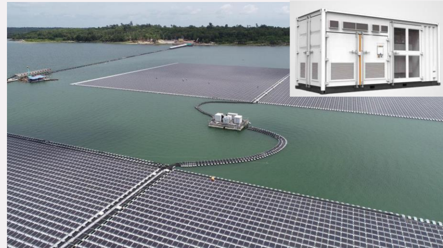
Thailand's Largest Floating PV Plant, 58.5 MW project in Sungrow supplied
