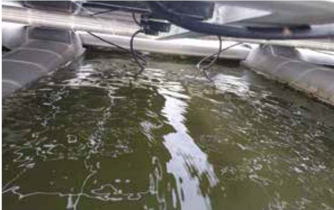
FIGURE 9.15 Connectors and cables submerged in water
